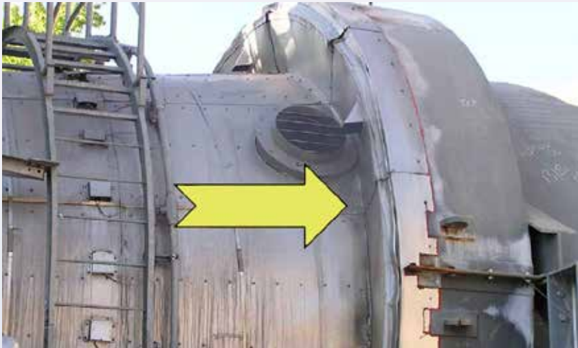
Corrosion and discoloration of the metal shroud is a key indicator of a failing Flex Seal
