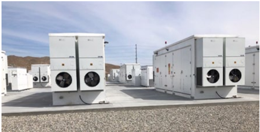
2. Redundant cooling systems are installed in each container to provide thermal management in the harsh desert environment
