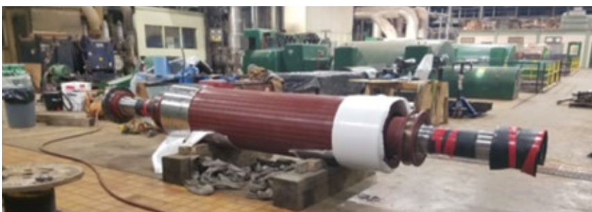
1. Generator rotor (field) awaits reinstallation following a shop rewind
