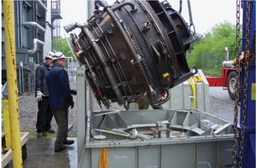
3. Low-pressure turbine is loaded into shipping container for trip to repair shop
