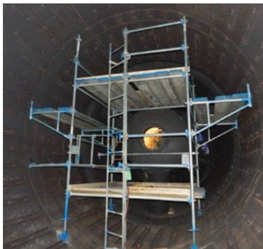
1. Diffuser-duct liner plates are supported by studs, ultimately attached to the casing
