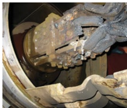
3. Failing flexible connection joint can be quite expensive to repair
