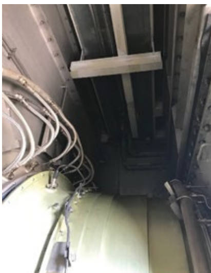
2. I-beam centered above the LPC allows case removal without extensive rigging
