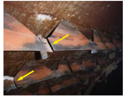
6. Cracked scallop bars will vibrate; studs will loosen or break free
