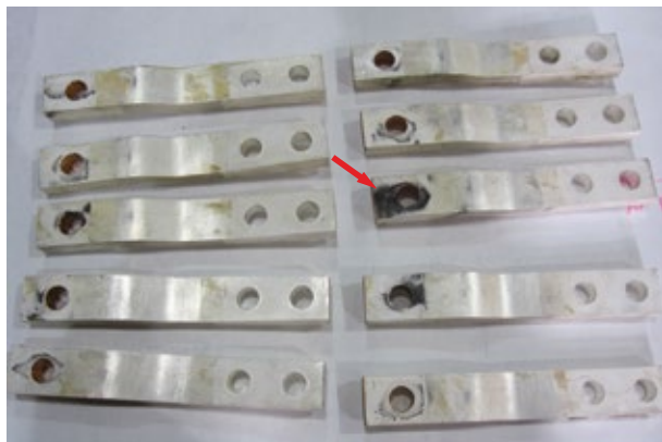
8. Black oxide residue indicates joint sparking at multiple single-bolt locations. Arrow indicates where most severe sparking occurred
