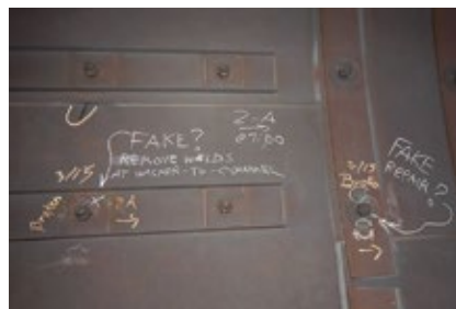
3. Some stud repairs can be cosmetic, not structural
