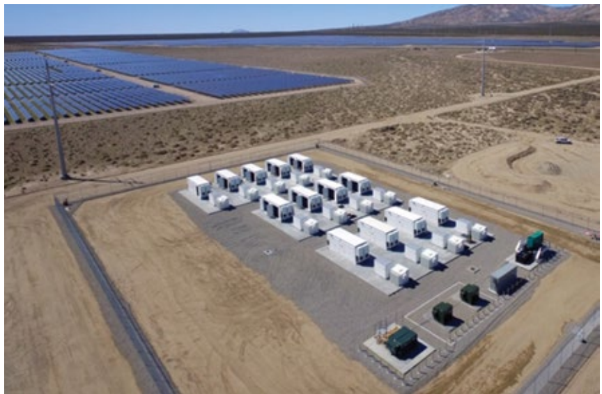
1. Ladwp's new BESS facility serves a huge solar PV area (with numerous wind turbines nearby) that will soon top 1 GW of capacity in California's Mojave desert
