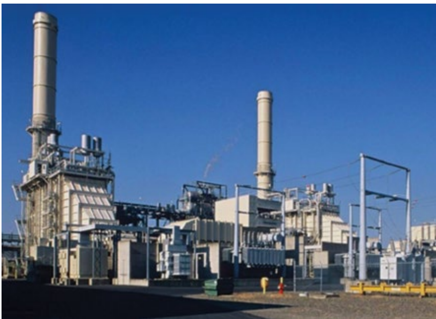
1. Puget Sound Energy Inc's Ferndale Generating Station, a 270-MW, 2 × 1 combined cycle powered by dual-fuel 7EA gas turbines, is operated by NAES Corp. The Ferndale (Wash) plant was built by a Tenaska Inc affiliate, commissioned in 1994, and sold to PSE in 2012
