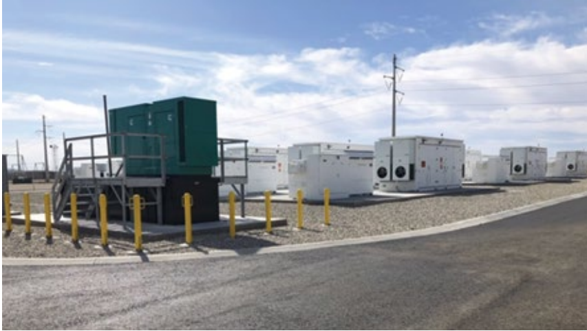
3. Thirteen battery/PCS containers make up LADWP's Beacon Solar BESS facility, one serving as a "spare." Backup engine/gen set in foreground (green structure) ensures cooling to the containers in the event of loss of grid power
