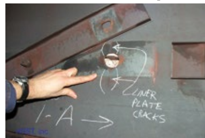
4. Liner cracks around the stud holes indicate long-term damage
