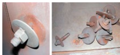
2. Loose or broken studs can indicate a deeper problem
