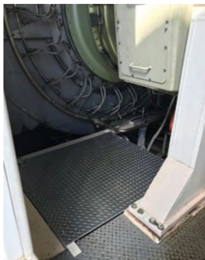
1. Installation of a custom platform eliminated the need for an extension ladder and fall protection
