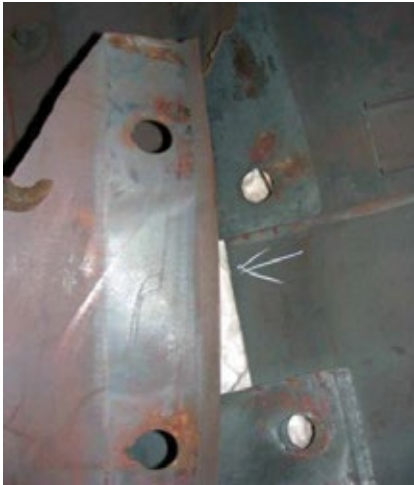
7. Exposed insulation can break free and foul tubes and catalyst
