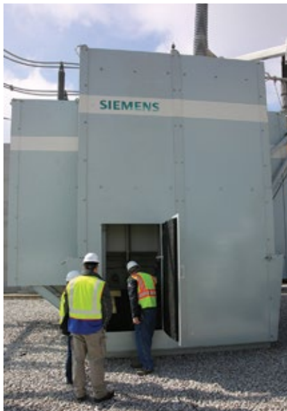
1. Doors provide access to control cabinets, pumps, fans, and other components requiring regular inspection and maintenance
