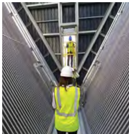
8. Narrow walkways are inherent in induced-draft units
