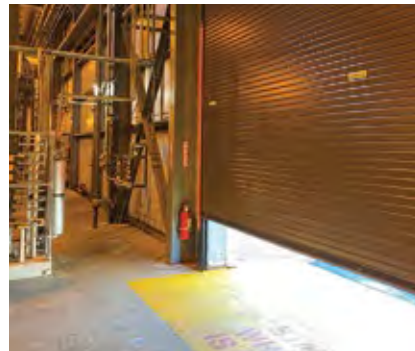
4. Red LED light strips signal when the overhead door is in motion
