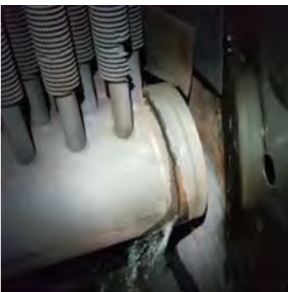
9. End-plate failure of header in the high-pressure superheater
