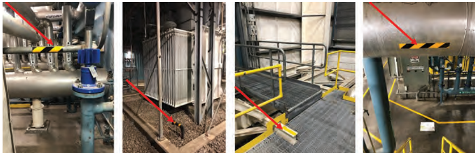
Trip and clearance hazards were mitigated by increasing awareness using appropriate signage
