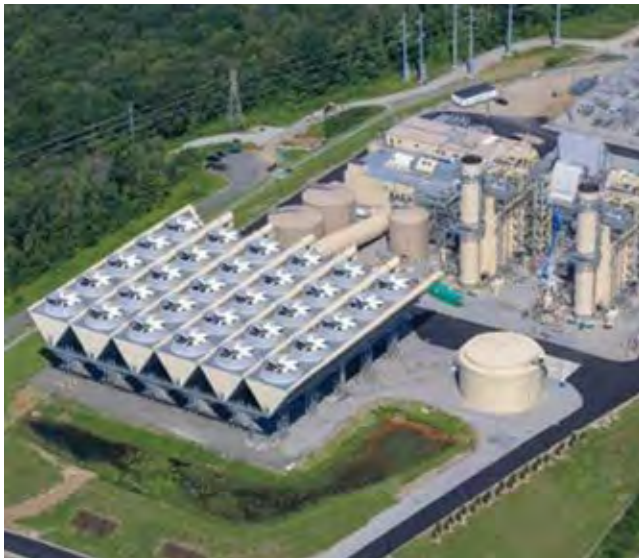
A. Induced-draft ACC at CPV Towantic Energy Center (left)
