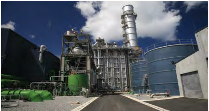
6. NewGen Power Kwinana is a 1 × 1 combined cycle with a 160-MW gas turbine, and 160-MW steam turbine that gets half its rated output when the HRSG is supplementary-fired
