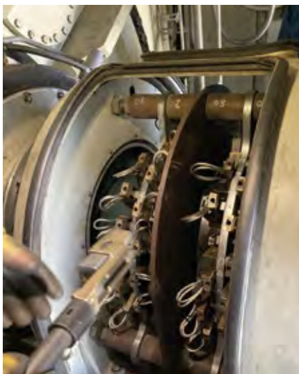
1. Technician inserts brush equipped with an insulated handle
