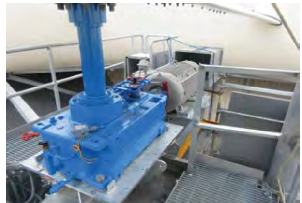
D. Each motor/gearbox assembly is 30 feet above the walkway (below)
