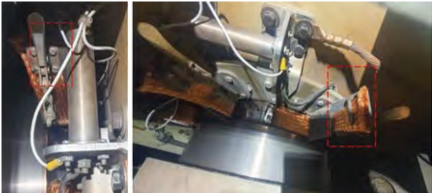
4. Braid fixing lever is at the left; grounding-system arrangement at right illustrates how simple it is to access the braid for maintenance and removal
