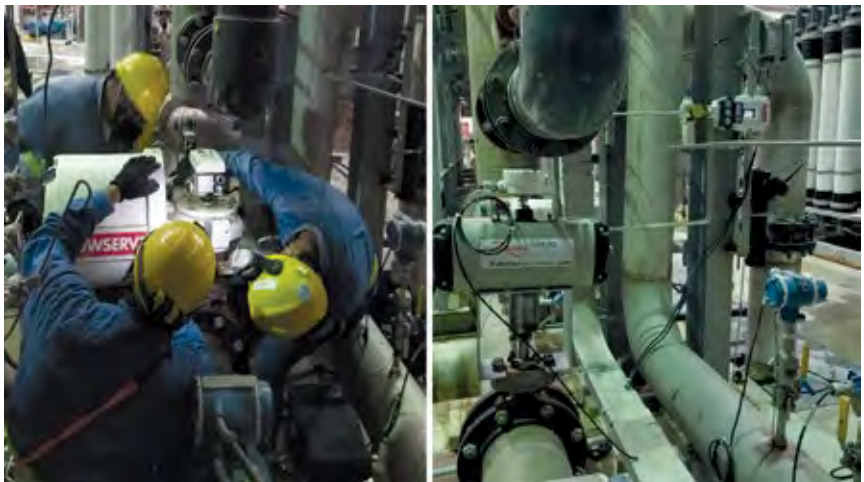
5. Original actuators for valves serving the ultrafiltration modules were replaced with smaller, lighter alternatives to improve maintenance access and mitigate ergonomic concerns
