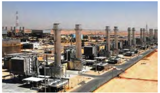
Riyadh 9 , a/k/a PP9, is a 1680-MW station with eight gas/diesel-fueled engines installed in 2004 and 20 crude/gas-fired units installed in 2007. All units are rated 60 MW
