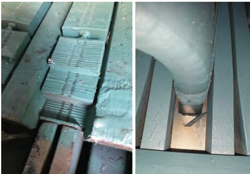
1. OSSB in Model 7FH2 and 324 generators can cause a unit to “go to ground,” experience a phase fault, and melt copper and iron
