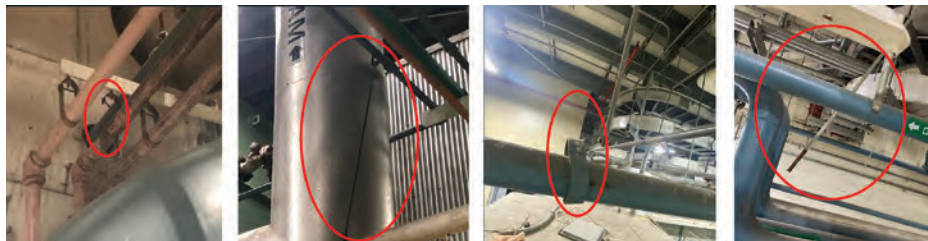
Piping-support failures and the possibility of falling objects. Broken pipe-support components were identified and fixed or replaced; hangers no longer providing the level support required were adjusted
