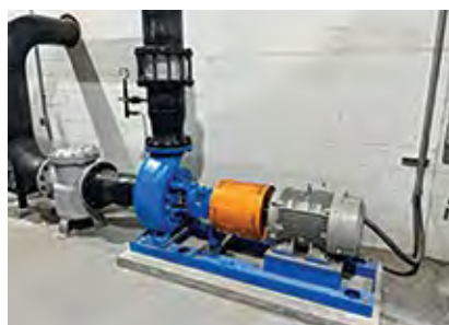
CCW pump with a 480-V driver in place of a 4160-V motor reduced power consumption by 70% when Rumford is offline
