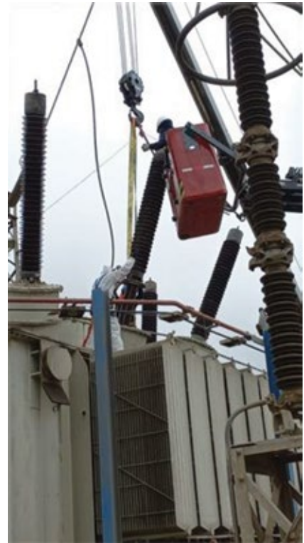
1. A bushing failure several years ago forced Ventanilla out of service
