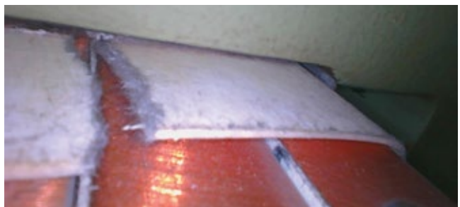
5. Failed/cracked slot liner was identified during bore-scope inspection (below)
