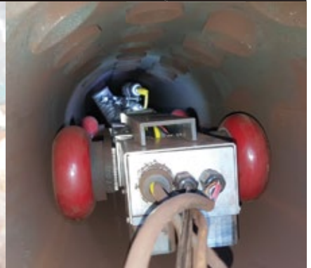
Internal Inspection, Collecting Tube Video & Measuring Wall Loss
