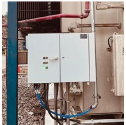
2. Online monitoring of critical transformer data helps identify issues before they cause an outage
