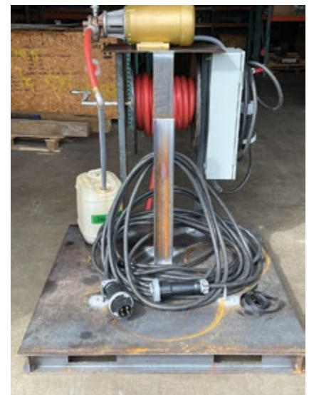
2. Cooling-tower tote, at ground level, eliminates the need to carry 40-lb pails of oil up and down the tower's stairs
