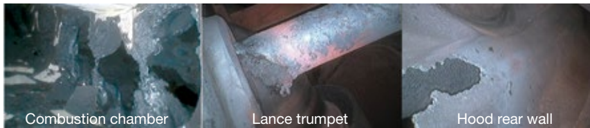
3. Damage to the Rocksavage combustor forced the unit out of service for six and a half months
