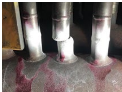
3. Failure in stainless-to-CSEF steel transition. EPRI is aware of steam leaks or failures in both link piping and tubing
