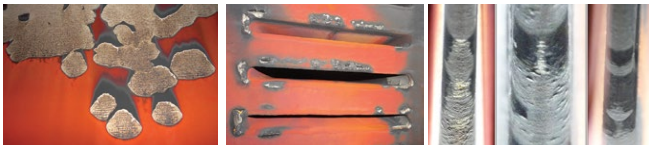
1-3. Metal loss from ACC duct walls attributed to LP-turbine steam exhaust (left); erosion/corrosion at ACC tube inlets (center) and 3 to 6 ft downstream of the tube inlets (right)
