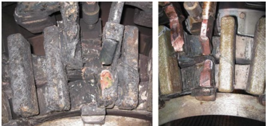
19. Generator endwinding resonance and main lead failure are among the leading stator issues
