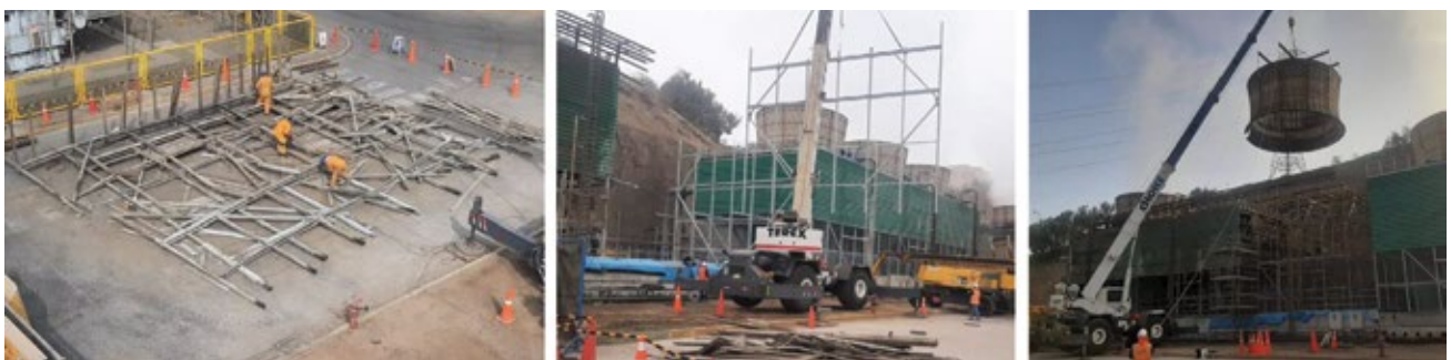
8. Tower 2 was disassembled (left) and reassembled (center) using glass-fiber reinforced plastic in place of wood for structural members. Fans were upgraded to increase air flow (right)
