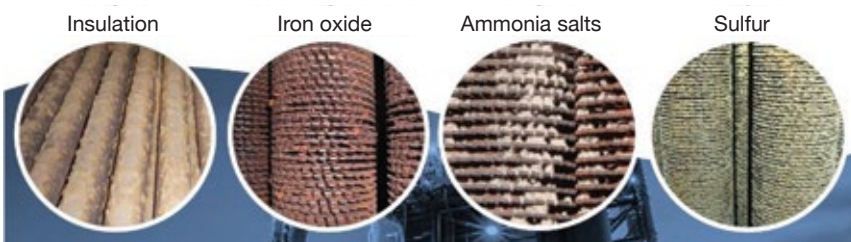
4. Types of fouling/deposits found on heat-transfer surfaces in Ventanilla’s HRSGs (l to r): insulation, iron oxide (rust), ammonia salts, and sulfur
