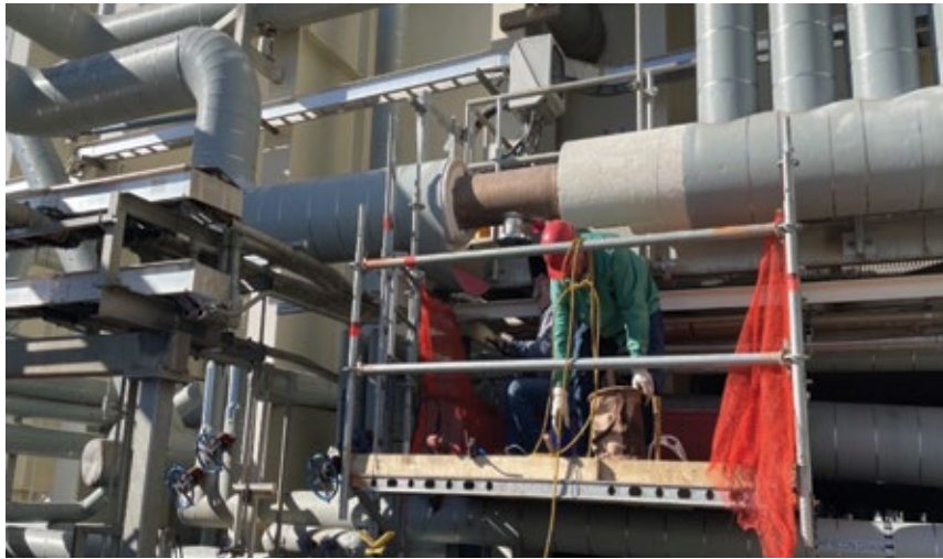
7. SCR piping is modified to allow connection of a vacuum truck for cleaning ammonia injection nozzles
