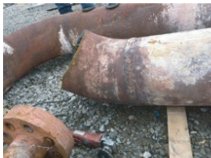
IAFD. Piping downstream of the attemperators may be the most highly fatigued piping in the powerplant
