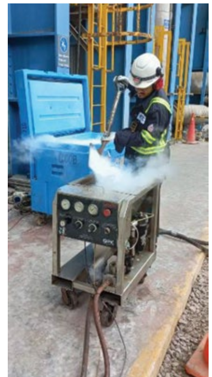
5. Dry ice was injected at ultra-high pressure to remove the fouling/deposits found in HRSG tube bundles
