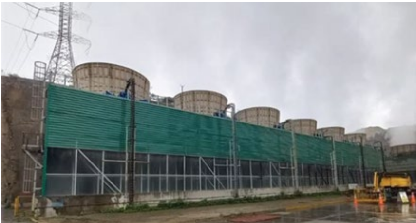
7. Ventanilla’s wet cooling towers each have six fans. Four fans remained in service throughout the overhaul activity
