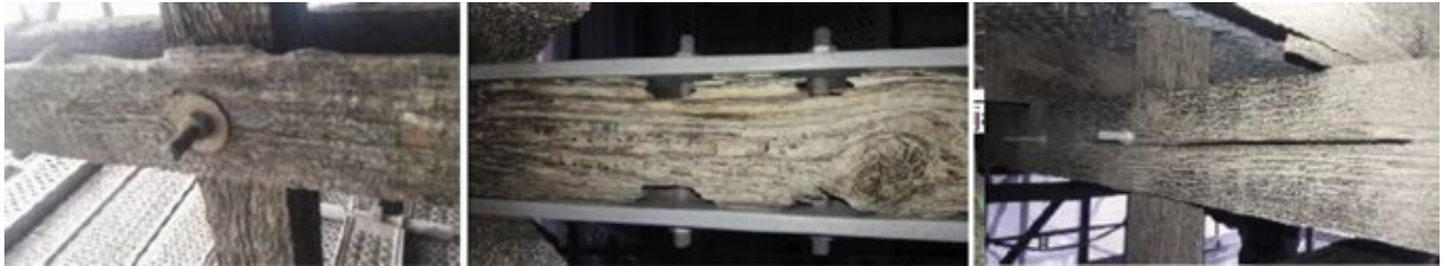
6. Cooling tower 2 was in poor condition. Examples: Loose tie bolts (left) and deterioration of (center) and fractured (right) structural members
