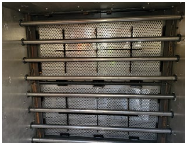
2. Ammonia distribution within the exhaust-gas cross section is a major factor in the catalyst's ability to properly reduce NO x levels
