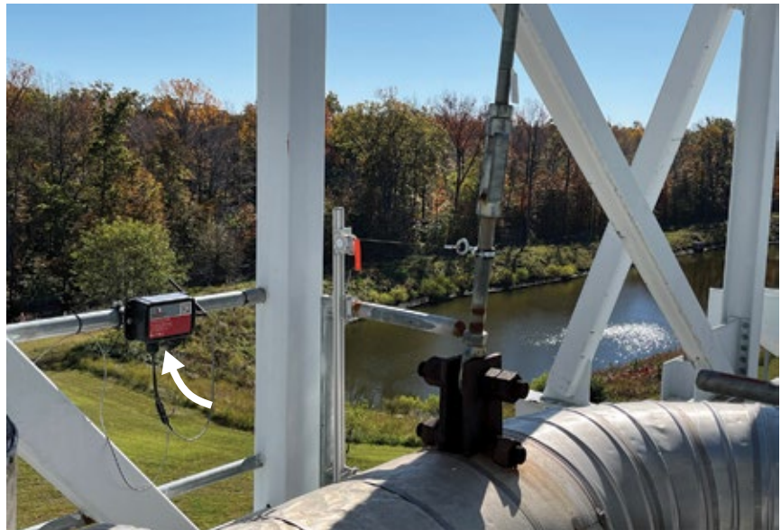
2. Pipe-hanger position monitor (arrow) helps predict high-stress locations within the piping system
