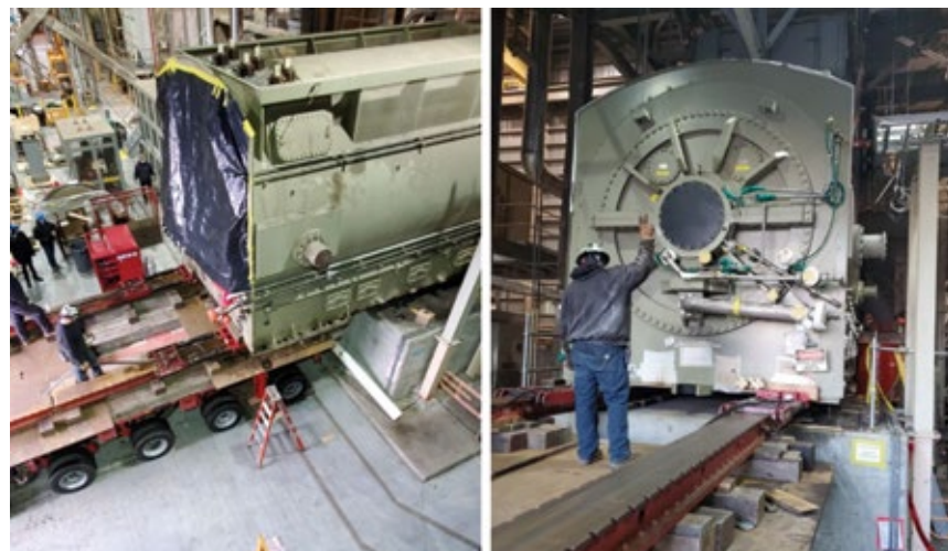
5. Complete stator replacement in two steps: Slide damaged stator off its foundation and onto a trailer (left) and slide new stator onto the foundation (right)
