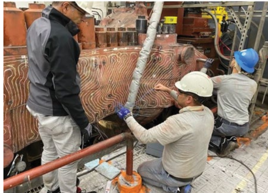
4. Steam-turbine warming dramatically reduces unit startup time. Here technicians install removable heating panels on the upper portion of the turbine casing
