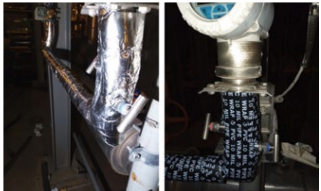
3. Thermal insulation prevented freeze-up of water-steam columns
