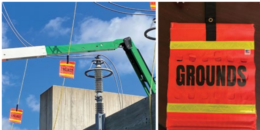
1. All-weather, high-visibility reflective flags draw attention to HV ground connections
