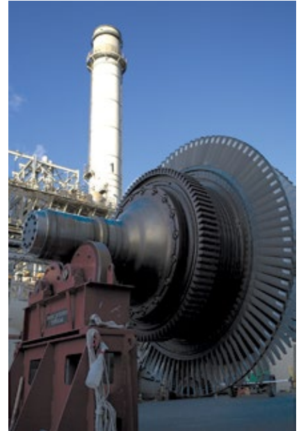
4. First-, second- and third-stage turbine buckets were replaced (Fig 3, left end of shaft)
