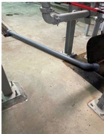
2. A section of CPVC was arranged with a union to permit easy assembly/disassembly for discharge to the filtrate sump
