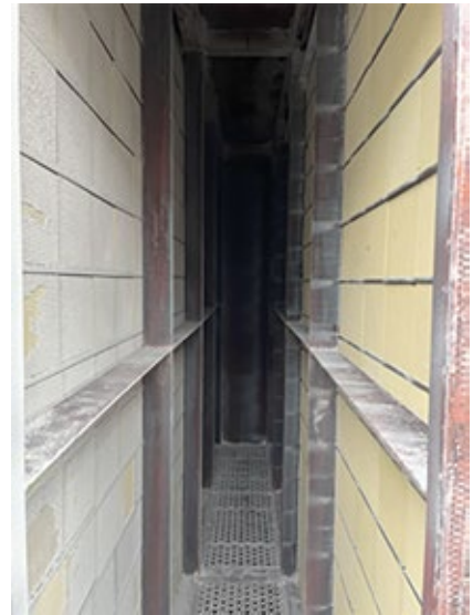
1. Inspect SCR catalyst at every outage to ensure the catalyst face is not blocked by rust or insulation
