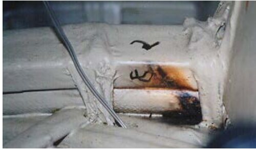
Figure 6-23. Arc Damage from Stator Hipot
