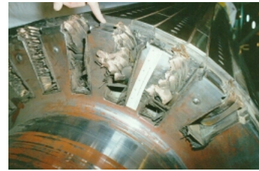
Figure 4-58. Open-circuited field. Root cause: 18/5 retaining ring fracture.
