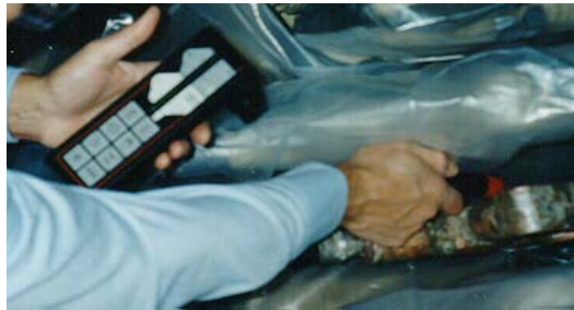
Figure 7-35. Checking for Stator Winding Leak using Halogen Gas Detector
