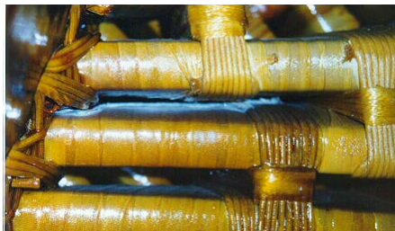
Figure 6-21a. Partial discharge at Line-to-Line Phase Break in Stator End Winding
