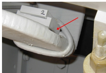
Figure 4-34. Bare copper exposed on a connection ring
