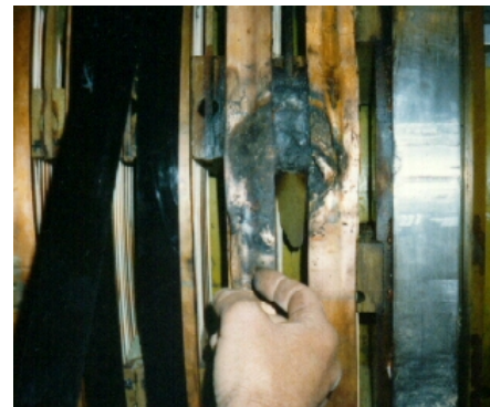
Photo 31. Two largest coils shorted together due to extensive contamination.
