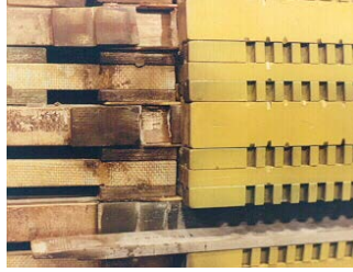
Figure 4-12. Broken Field Slot Top Creepage Block
