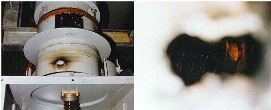
Figure 6-74 & Figure 6-75. Hole Burned in Isophase by Standoff Insulator Failure, External View and View of Insulator Through Hole in Cover.
