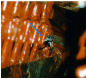
Figure 4-30. Broken braze on one seventh of a top-to-bottom bar connection
