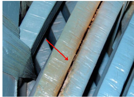
Figure 4-40. Heavy PD indications at a line-to-line phase break
