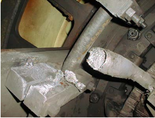
Figure 4-28. Burned connection ring. Note missing 10” of burned away lead.
