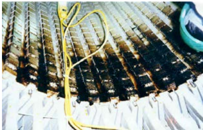
Figure 4-35. Severe bar vibration only at the ends of the core
