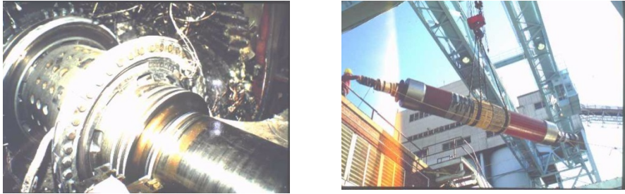
Figure 8-2 & Figure 8-3. Results of Retaining Ring Burst: Extensive Generator Damage and Replacement Field
