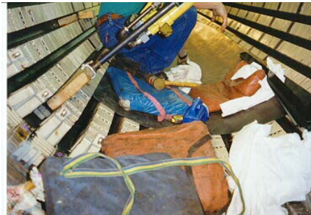
Figure 8-9. Stator Rewedging Equipment
