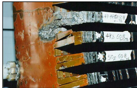
Figure 3-5. Core Damage Resulting from Over-fluxing
