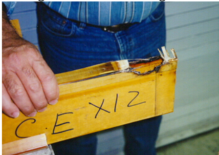
Photo 13. Slot liner with damage from an electrical creepage failure.
