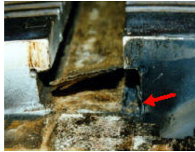
Figure 4-55. Forging burn due to double field winding ground. Root cause: old, worn-out insulation
