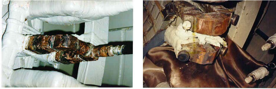
Figure 8-22 & Figure 8-23. Insulation Stripped from Direct and Indirect Cooled Series Loops (General Electric)
