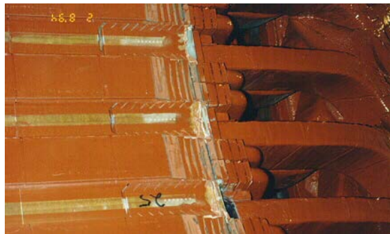
Figure 6-4. Damage from Contact Between Field and Stator Core
