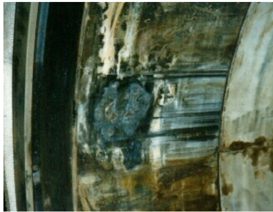
Figure 5-28 & Figure 5-29. Arc damage from shorting between 2 coils and resulting near-fatal burn damage to the retaining ring inside diameter.
