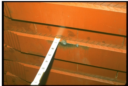
Figure 4-6. Core Damage from Small Object Impact
