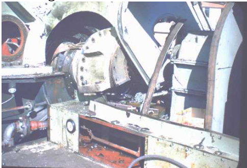
Photo 39. Non-drive end of the generator after forging failure.
