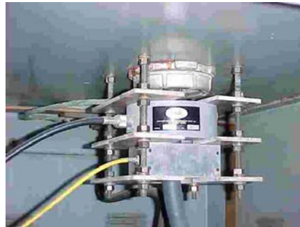
Figure 5-21. Two Radio Frequency Current Transformers Assembled on Lead to Neutral Grounding Transformer
