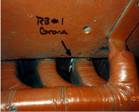
Photo 4. Burning at the junction of grading/grounding systems.
