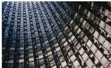
Figure 6-28. Heavily Contaminated Stator Core
