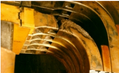
Figure 4-56. Fractured turn. Root cause: Braze location, reduced copper area, stress risers.
