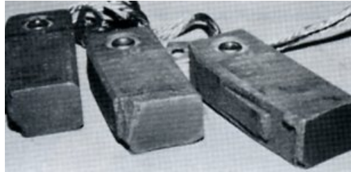
Figure 2-44. Chipped and ridged brushes
