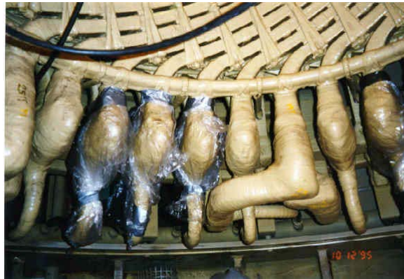
Figure 2-29. General Electric Taped Insulation (with 3 Loops Prepared for Leak Test)
