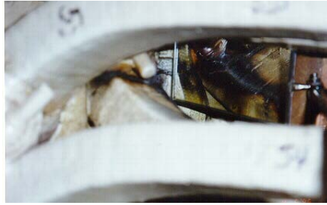
Figure 6-1. Arcing Damage from Hipot Test
