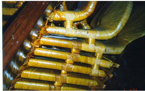
Figure 8-24. Partial discharge Degradation and Deposit in an Air Cooled Stator End Winding
