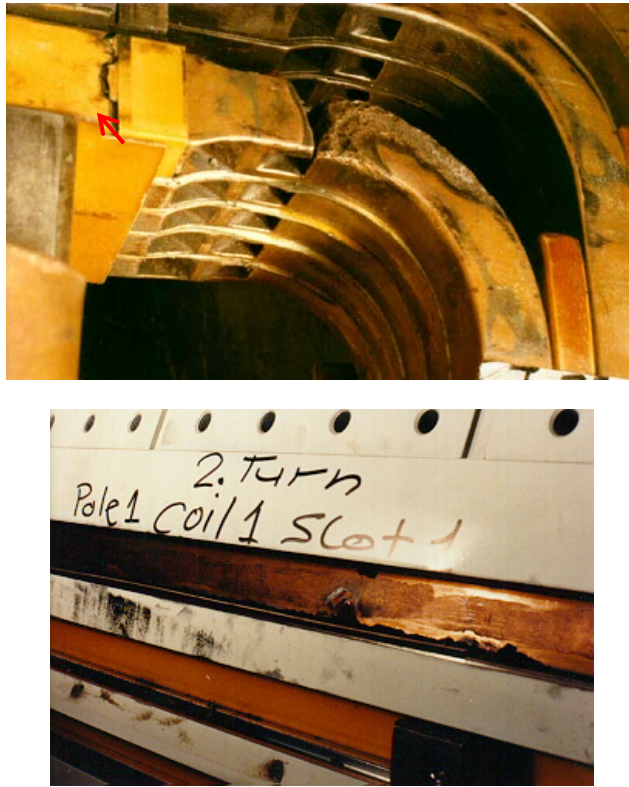
Figure 5-26 & Figure 5-27. Broken top turn and forging arc damage resulting from the break.
