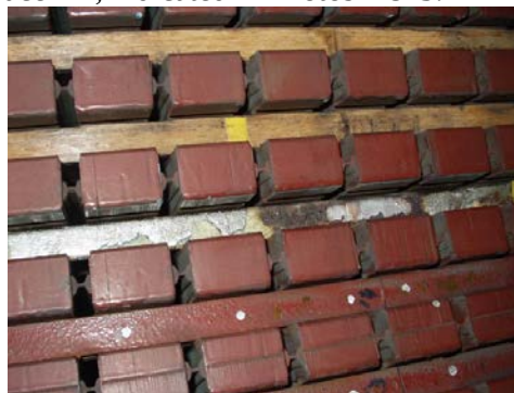
Photo 2. Significant surface partial discharge indication in the slot.
