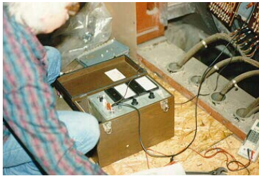
Figure 7-23. Instrumentation Measuring RTD Insulation Resistance
