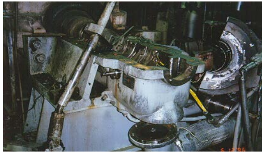
Figure 3-7. Broken Turbine Control Standard after Severe Vibration and Fire
