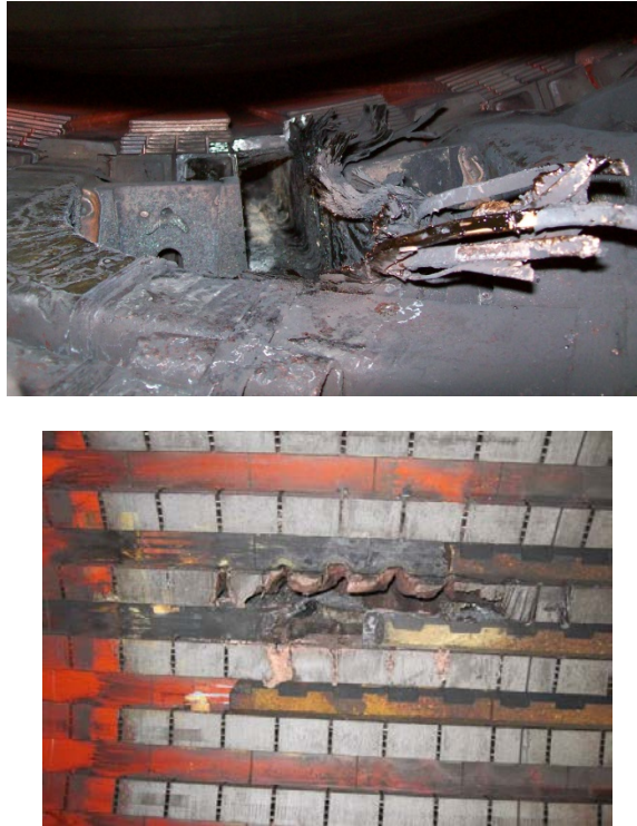
Figure 5-30 & Figure 5-31. Typical core and winding damage resulting from broken stator winding conductor.
