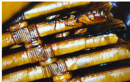
Figure 8-25. Deposit of Oil Decomposition Products in the Partial discharge Field of and Air Cooled Stator End Winding
