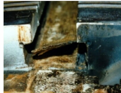
Photo 11. Failed asbestos-mica field slot liner.
