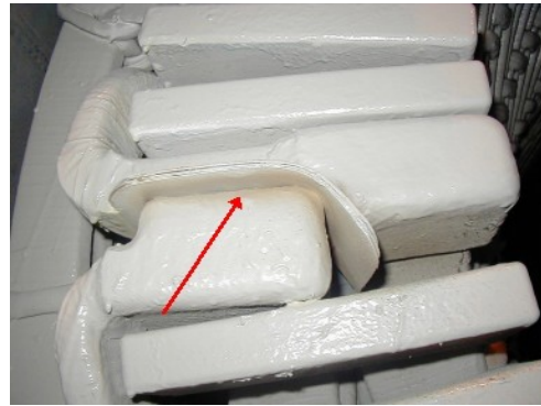
Figure 4-42. PD at a non-failed phase connection location
