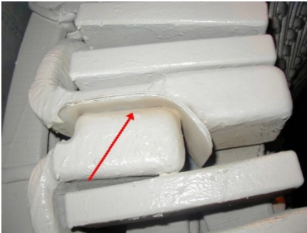
Photo 5. Indications of PD on the surface of one of the 3 line-to-line voltage phase break locations.
