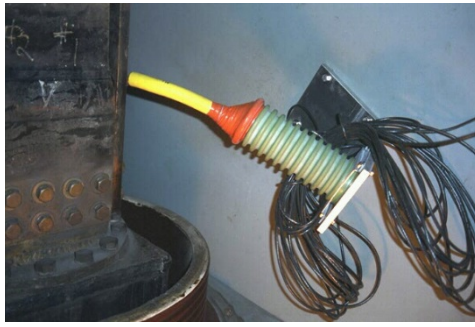
Figure 5-16. Line Pickup, 80 pF, with Cable not yet Connected (Iris Power Engineering)
