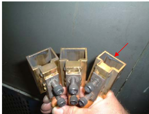
Figure 2-46. Carbon build-up inside brush box. (Cutsworth Products/Services)
