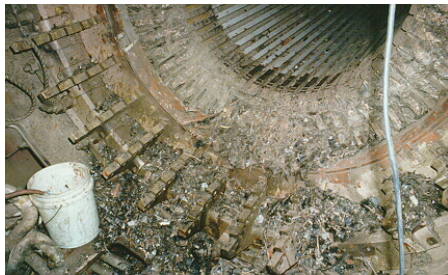
Photo 42. Damage to stator from ring failure.
