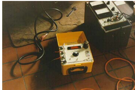
Figure 7-22. Digital Low Resistance Ohmmeter (DLRO) on the Left, and Megohmmeter to the Right.
