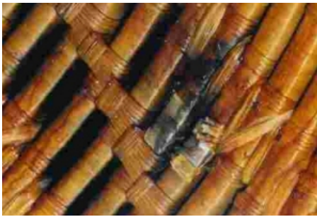
Figure 4-32. Arc damage from a short circuit between adjacent bars in an endwinding
