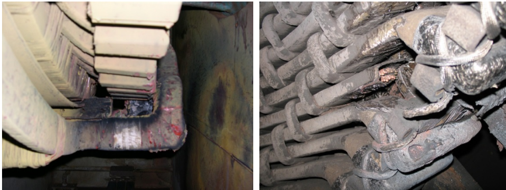
Figure 5-33 & Figure 5-34. Failed phase and series connection.
