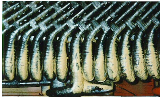
Figure 4-19. Foreign Material Deposit on End Winding from Cooler Leak
