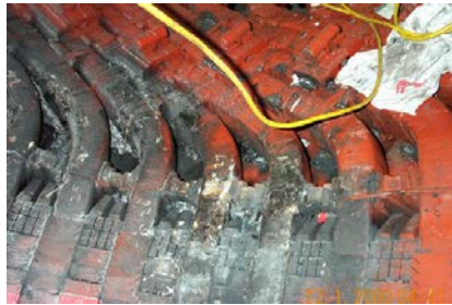
Figure 4-7. Complete Core Melt-down due to Lamination Insulation Failure.
