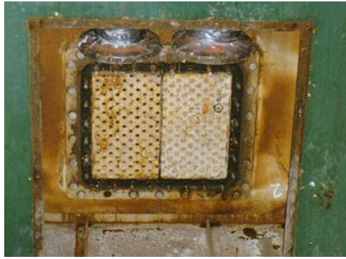
Figure 6-73. Cooler Tube Sheet with Cover Removed
