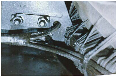
Figure 7-9. Stator Winding Support and RTD Cable After Internal Fire Ignited by High Potential Test
