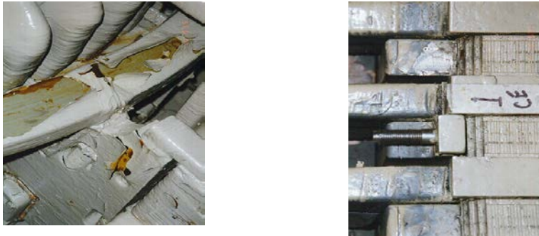
Figure 6-58 & Figure 6-59. Blistered Paint and Extended Armature Bars from Severe Over-temperature Incident
