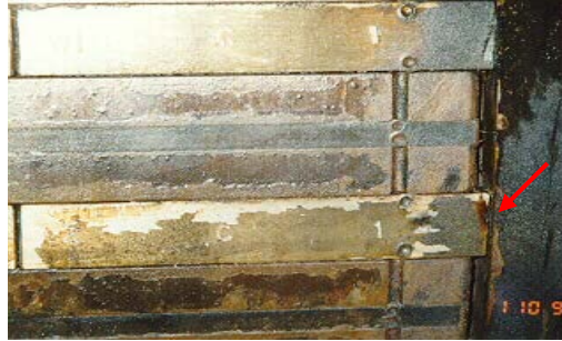
Figure 6-62. Field Wedge with Poor Lock and Axial Movement
