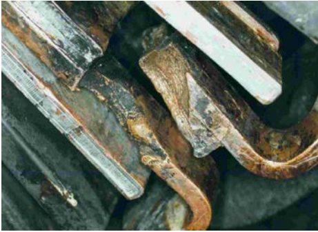
Figure 4-41. Failed connection after removing insulation
