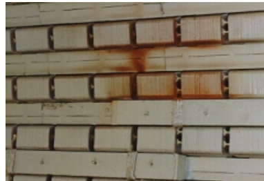
Figure 4-36. Wedge vibration on hydrogen-cooled generator
