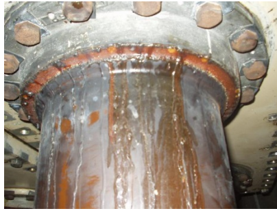
Figure 6-41. Flow of Sealing Compound through Failed High Voltage Bushing Flange
