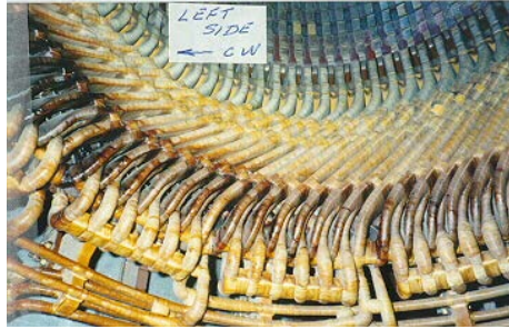
Figure 4-10. Stator Winding Failure from Inadequate Ventilation Design
