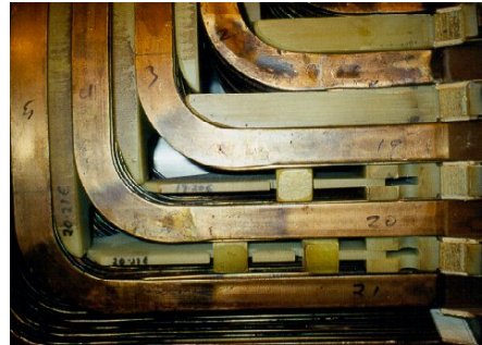
Photo 14. Insulating blocks used to insulate between coils by maintaining physical spacing.
