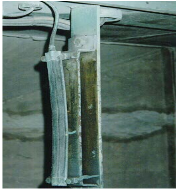
Figure 6-47. RTD Damaged by Careless Personnel
