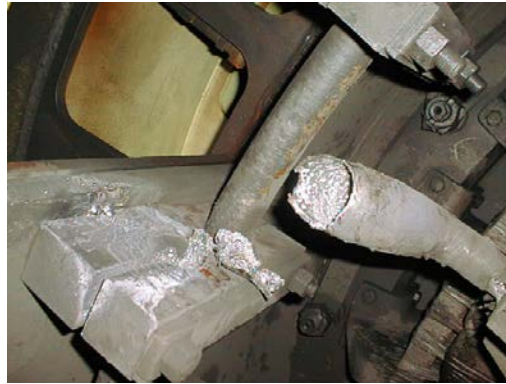
Figure 5-32. Burned away copper of a fractured connection ring.
