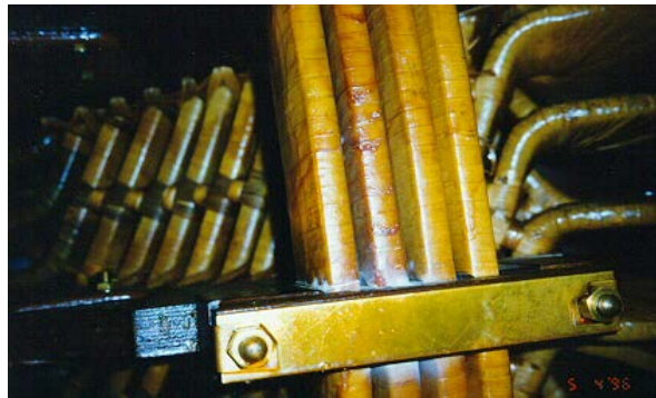
Figure 2-25. Connection Ring Support, with Vibration Activity.
