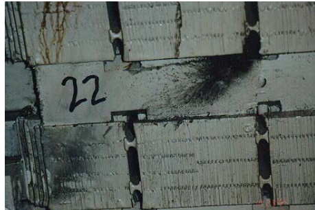
Figure 6-2. Dust Deposit on Stator Core Bore from Bar Vibration
