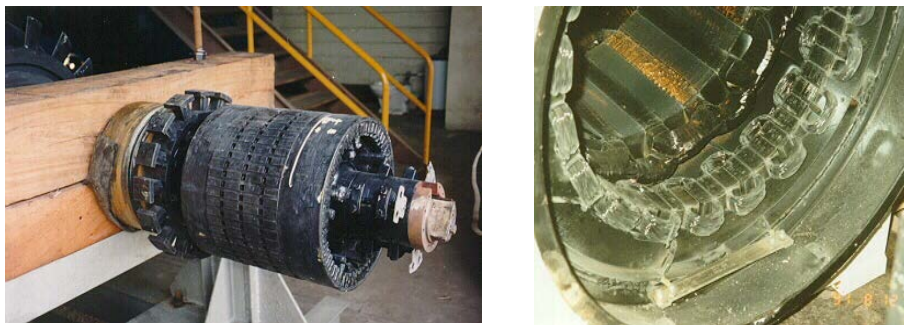
Figure 6-65 & Figure 6-66. Contaminated Shaft Driven Brushless Exciter Rotor and Stator
