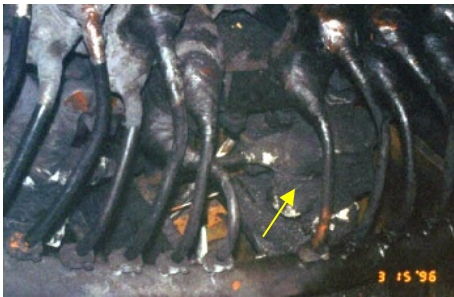
Photo 25. Series connection broken off and lying under winding.
