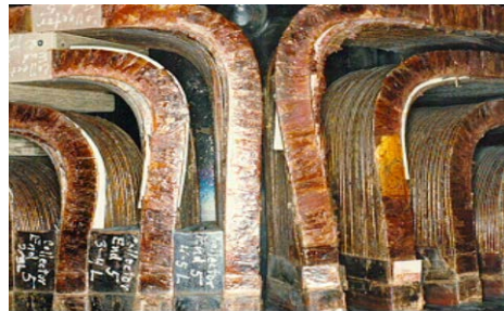
Figure 6-50. Field Winding Turn Distortion Accessible After Retaining Ring Removal
