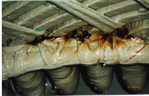
Figure 2-20. Evidence of Localized End Winding Vibration
