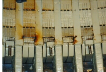
Figure 4-48. Grease generation from either bar vibration or core looseness
