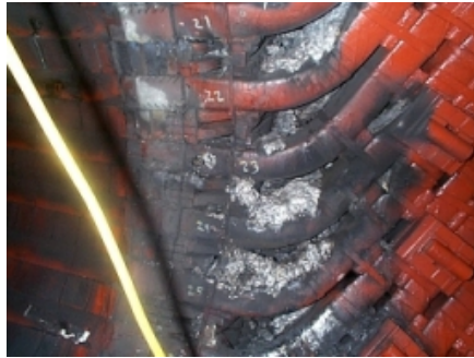
Figure 4-51. Melted core iron deposited in the stator endwinding
