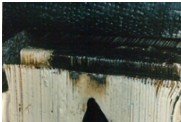
Figure 4-49. Local core lamination burning, probably due to minor core damage
