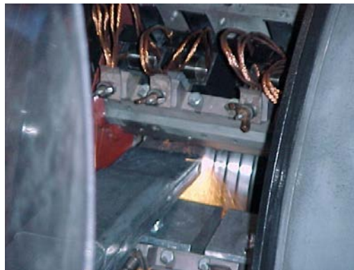
Figure 8-45. Stoning of large collector. (Cutsworth Products/Services)
