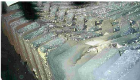
Photo 6. Failure at another of the phase break locations.
