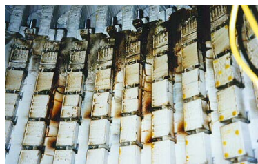
Figure 6-15. Severe “Greasing” Due to Bar Vibration at Ends of Core
