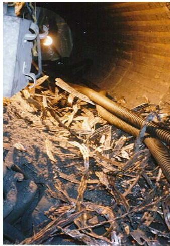
Figure 2-35. Residue of Stator and Field Windings after 3-phase Breaker Closure with Generator at Standstill.
