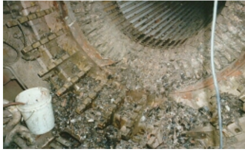
Figure 4-62. Stator winding after retaining ring burst. Note that the bars are still in the slots. (The stator winding has not been removed.)
