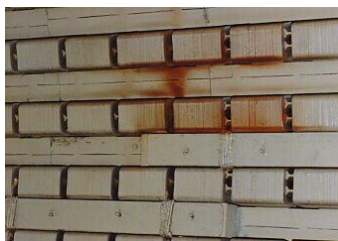
Figure 8-10. Red Dust Generation Resulting from Wedge Vibration in the Stator Slot Dovetail
