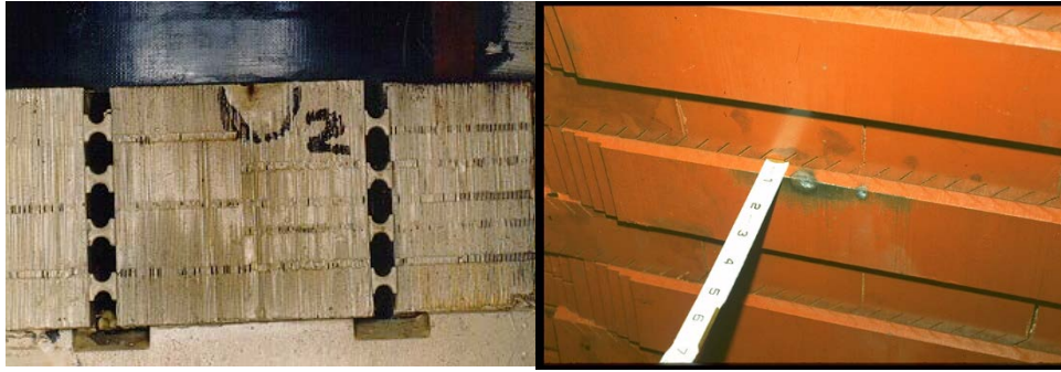
Figure 6-29 & Figure 6-30. Minor Core Burning Probably only Requiring Small Amounts of Grinding and/or Etching to Correct
