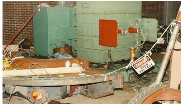
Figure 7-3. 60Hz High potential Transformer
