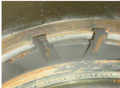
Figure 6-61. Rust Accumulation on Centering Ring and Retaining Ring
