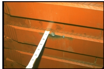
Figure 4-50. Broad heating pattern, probably from lamination insulation failure
