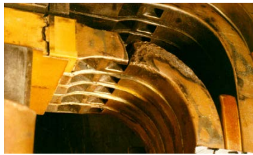
Figure 4-13. Arc Damage to Copper Conductors from Broken Top Turn
