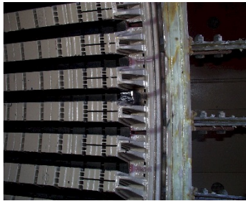
Figure 8-31. Core Damage and Burning of Iron at Bottom of Slot
