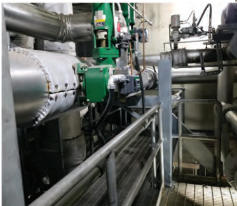
Ducting installed to send heated air from turbine enclosure to inlet, preventing icing at bell mouth and IGVs
