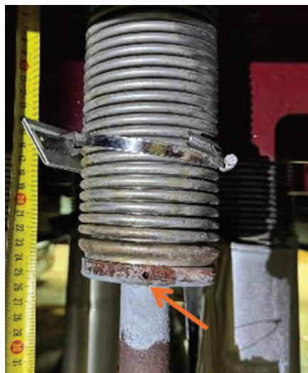
9. HP economizer drain tube leak
