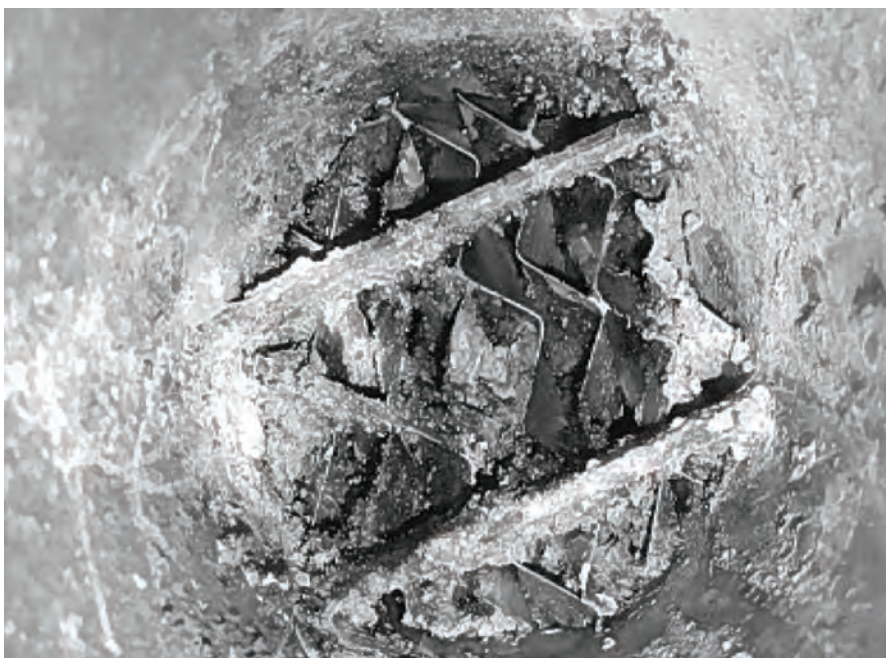
Vector Systems. Poor ammonia purity introduces contaminants that corrode AIG internals, form salts, and degrade SCR catalyst performance and longevity
