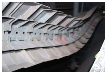
6. Failed duct burner
