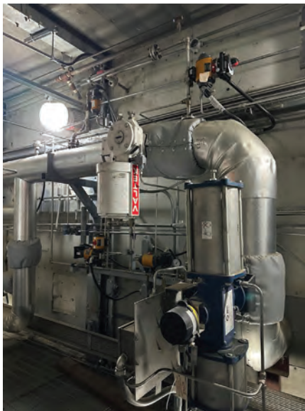
Purge credit upgrade reduces start-up time and HRSG thermal stress while improving package durability through new logic and valve modifications
