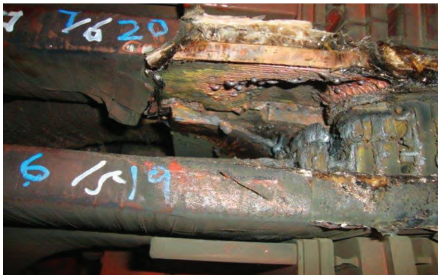
National Electric Coil. AEROPAC II generators can experience stator winding failures near the core exit from endwinding looseness, harmonics, and insulation degradation
