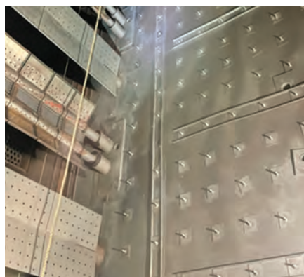
5. No sidewall impingement after 16 months, Gemini duct burners
