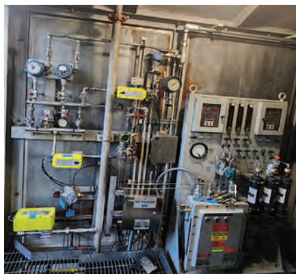
1. Operator-initiated purge enhancements. Remote range-change analyzers, MOV isolation, and interlocked sequencing replace variable manual steps with a verified process
