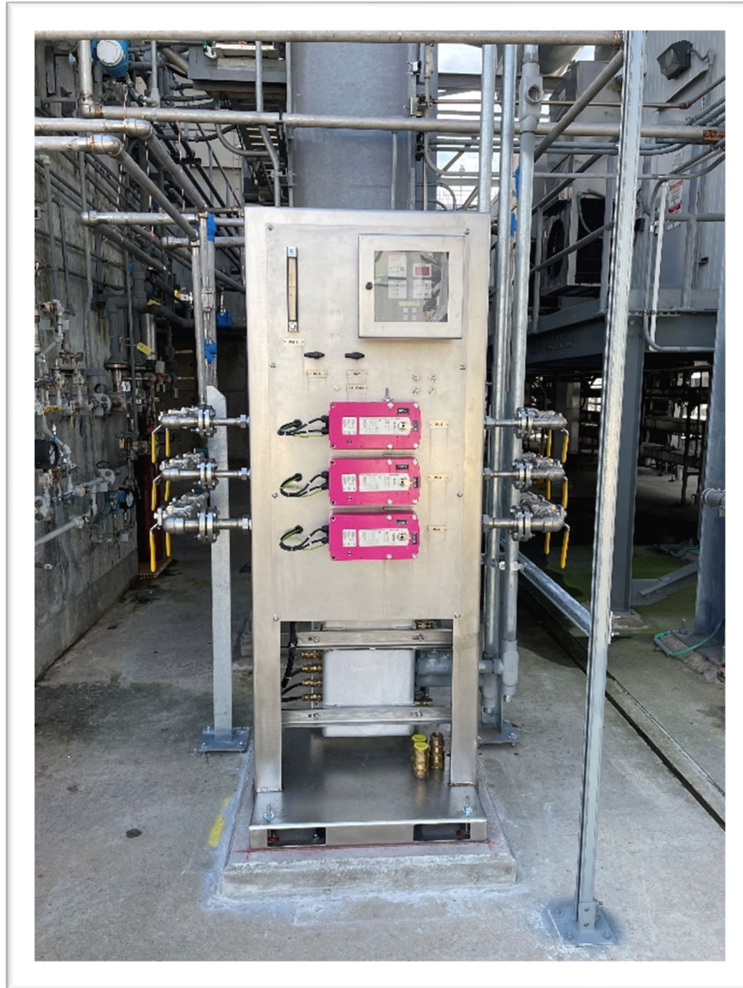
Remote Automation Panel
