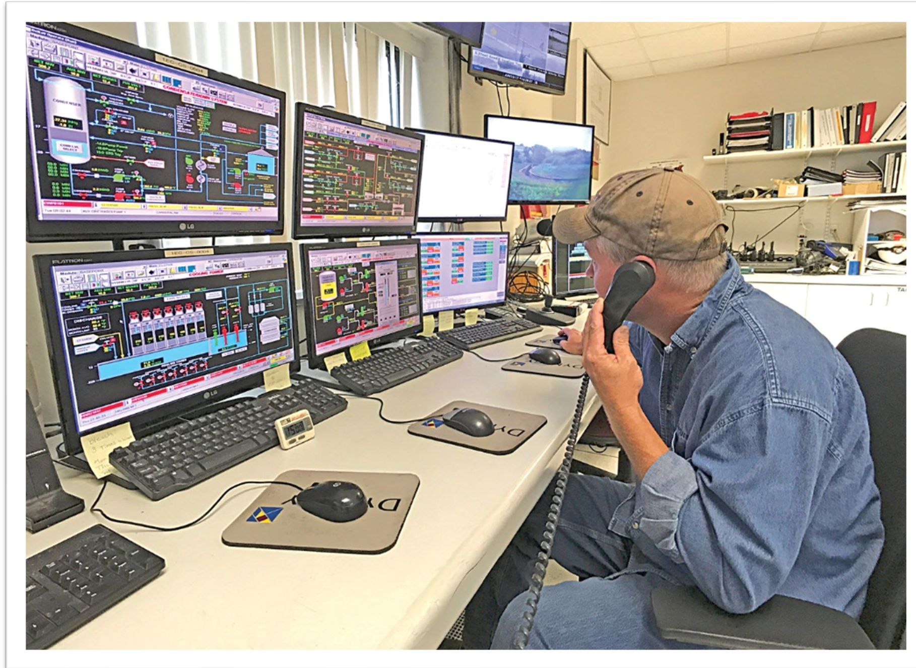
Operator-Initiated Automated Generator Purge
