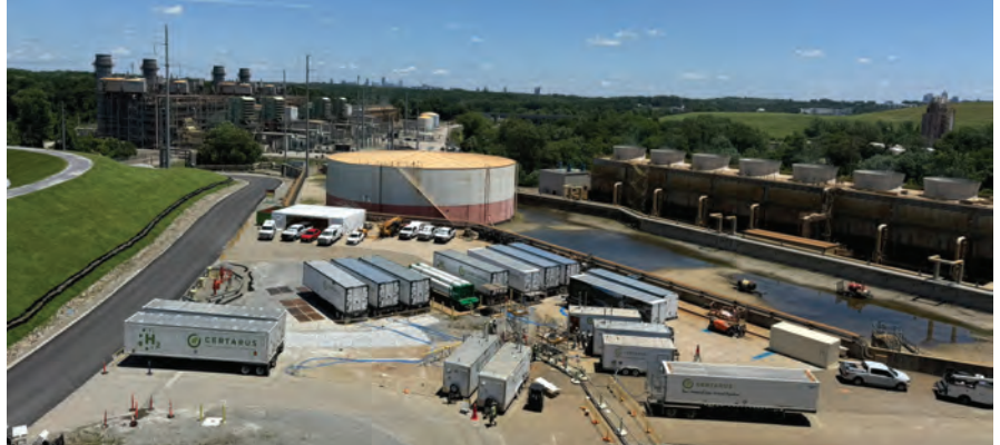
Hydrogen storage and delivery system
