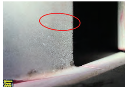
3. Stator Row 0 vane 34 exhibits significant crack which could have wiped out the machine if liberated. User urges others to perform TIL1509
