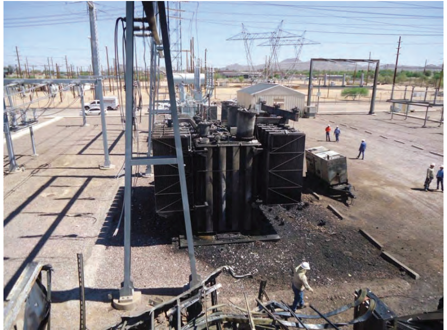
The worst-case scenario. Proactive transformer monitoring, testing, and maintenance can greatly reduce the risk of a catastrophic loss
