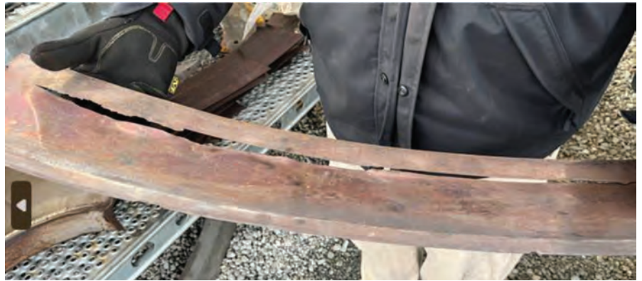
6. Condition of exhaust flex seal and replacement was one of several unexpected findings during site compressor modernization project
