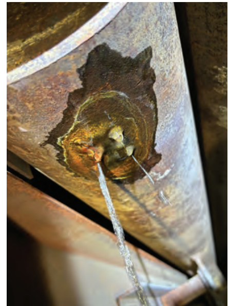
7. HP evaporator header failure
