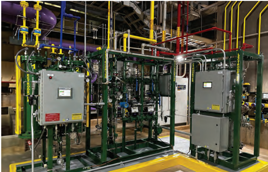
Lectrodryer: Automated generator purge and H2 dryer package can be integrated with OEM H2 piping, reduces purge duration from up to half a day to less than an hour, and is initiated by control room operator or at the local HMI
