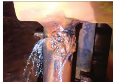
10. Pad weld leak in LP evaporator
