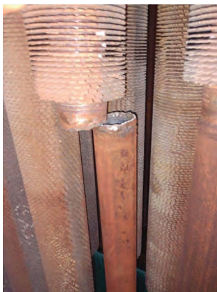
3. LP preheater damage at Midland
