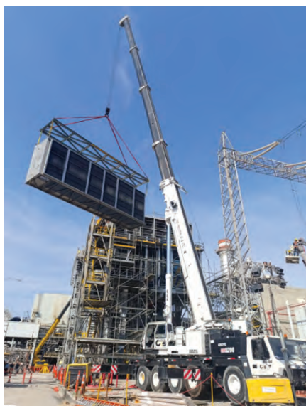
4. Crews lift and position new stainless filter-house modules following removal of existing filter, pre-filter, and evaporative-section components
