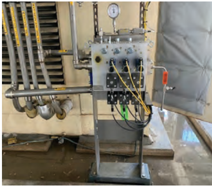
8. Seals failed in all six dump valves of the trip manifold assembly during a controls modernization; prelim RCA suggested design/manufacturing defect allowing excessive travel of the poppets
