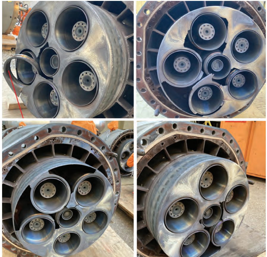
1. Combustor flow sleeve experienced potentially catastrophic damage from less than 10 minutes of combustion dynamics at 25 psi/170 Hz as a result of a control malfunction
