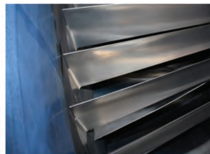
4500 hrs since last wash using E12 filters
