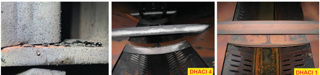
3. Two recurring field lessons from FFS programs: (1) gel-like deposits (“gunk”) have been documented (left) in LP drums when products are applied without an up-front Section 8 review, and (2) ACC two-phase FAC (middle) can show improvement in some cases, evidenced by reduced DHACI and lower condensate iron (right), but many plants see little to no arrest, so claims of universal ACC benefit should be treated cautiously
