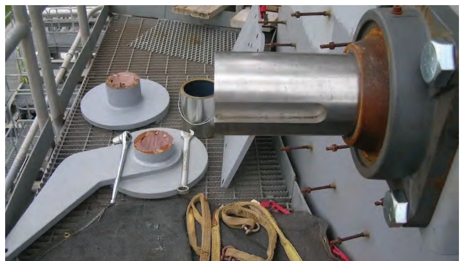
Outage inspection focuses on root causes , checking actuator performance, blade alignment, and shell-contact witness marks; early fixes prevent repeat failures, start delays, and safety risks.
