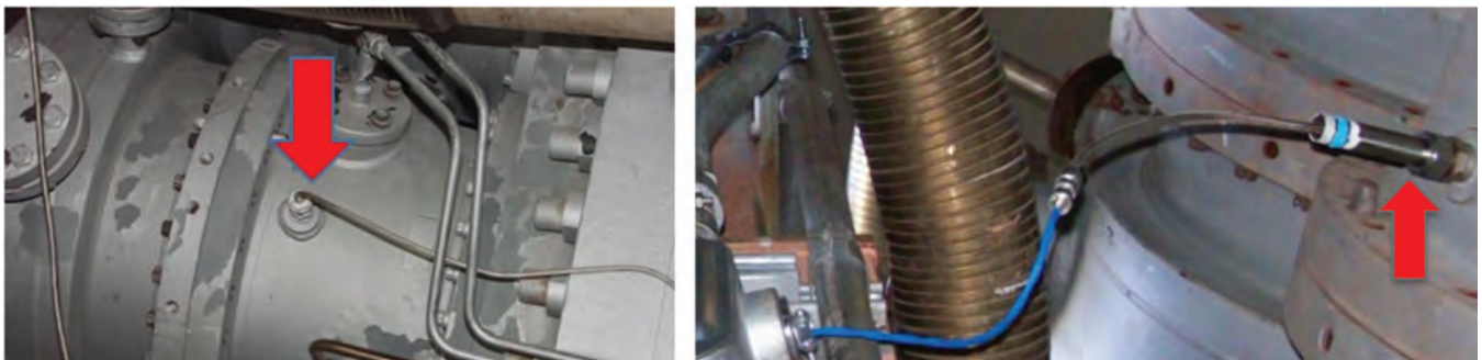
1. A useful GEV 7FA comparison: legacy tube-mounted hardware feeding a purge box versus a direct-mounted high-temperature sensor installed on the combustor housing
