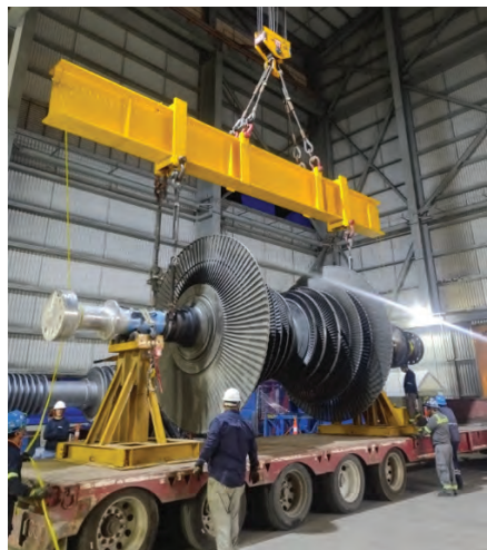
2. Steam turbine work included center-line readings, front-standard foundation review, HP-IP rotor preparation, LP rotor installation, and steam valve maintenance
