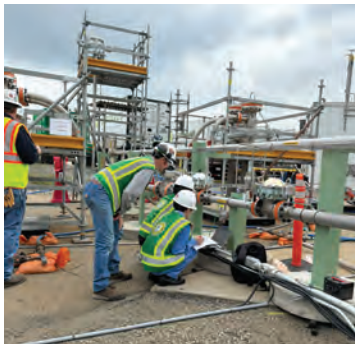
Testing of worker and monitor regulating valves
