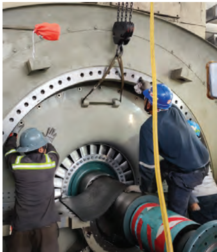
1. Finishing touches on rotor replacement, component upgrades, generator electrical testing, combustion assembly, and unit closeout
