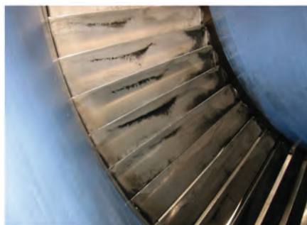
1200 hrs since last wash using F8 filters
