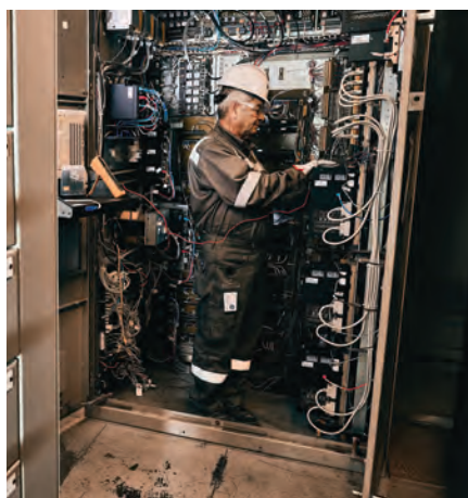
Controls. Build operational expertise through hands-on control system training and diagnostics
