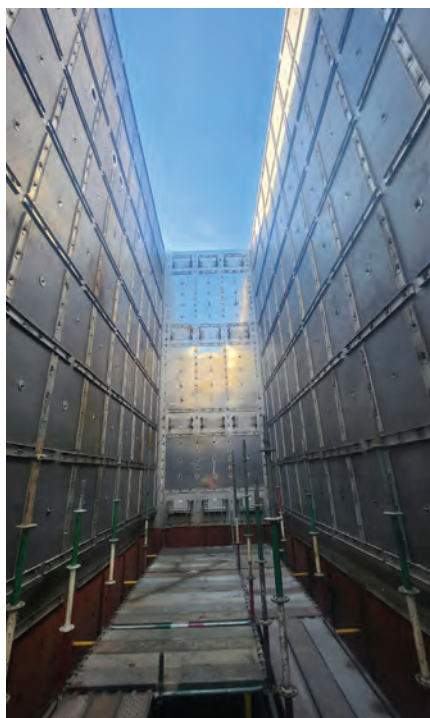
2. Interior of a 501D rectangular exhaust stack with a floating liner system
