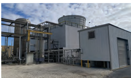
9. New cooling towers at SLEC
