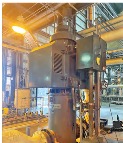
1. Condensate extraction pump
