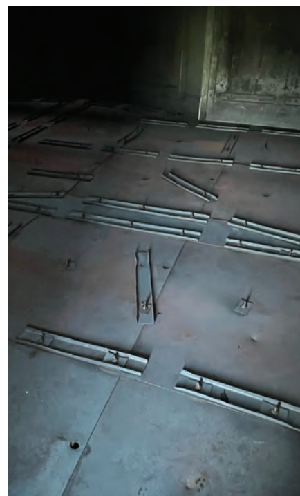
3. Damaged exhaust-liner sheets with deformed or detached batten channels
