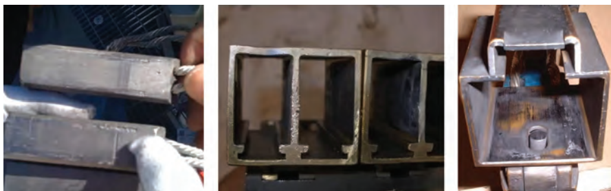
1. Carbon deposits, dirty conditions, holder damage, or poor tolerances can restrict brush travel. With only 3 to 5 lb of spring pressure, even minor binding can compromise brush-to-ring contact, leading to arcing, chatter, and escalating collector-ring damage
