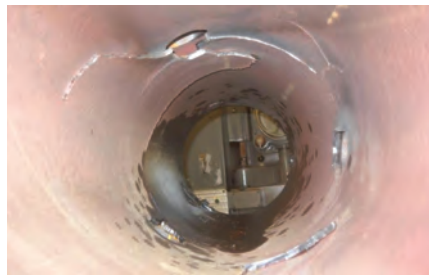
2. Attemperator failure resulting from thermal shock
