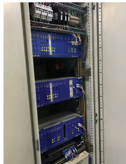
4. Alstom BlueLine gas turbine controls
