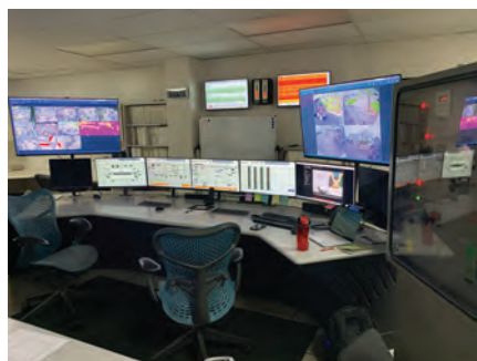
5. The control room at SLEC
