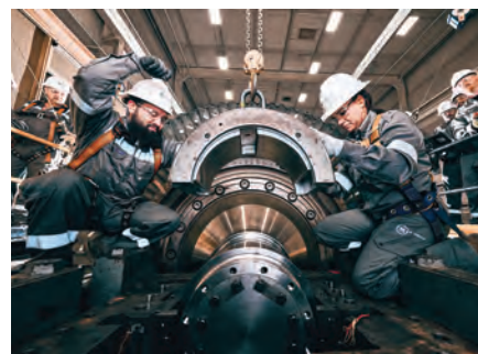
Generator. Experience generator technology up close through practical, hands-on training
