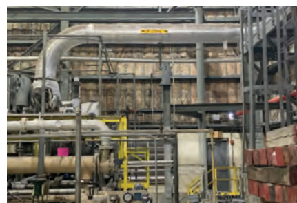
6. The HP steam line between the HRSG and the steam turbine
