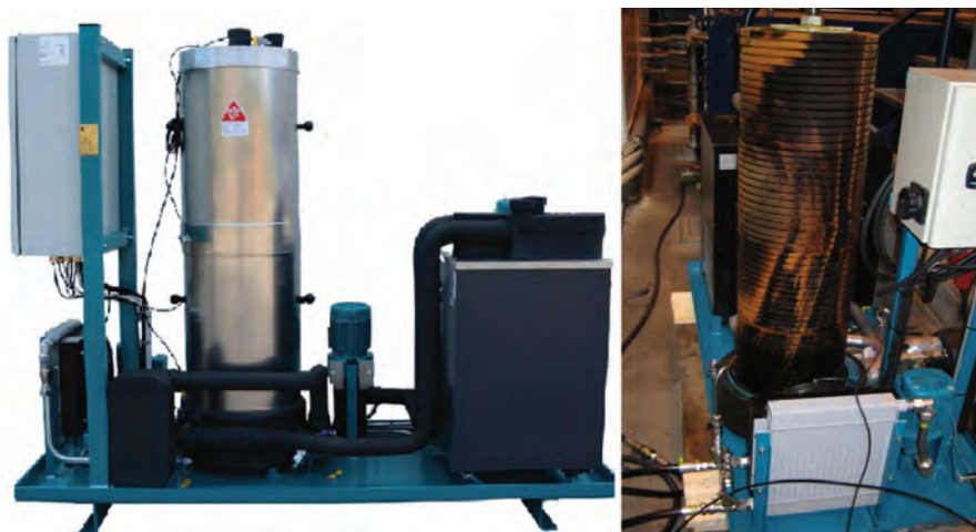
3. An off-line varnish-removal unit draws oil from the bottom of the reservoir and returns conditioned oil at the top, removing dissolved varnish during operation and settled contamination during outages
