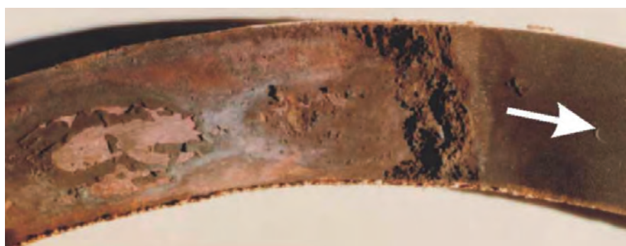
2. Oxide flaked from a hollow conductor and redeposited downstream in a bend after poor operation and layup
