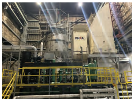
3. Vertical combustor sits above the gas turbine, inlet air in cream on right, and the lube oil system in green in front
